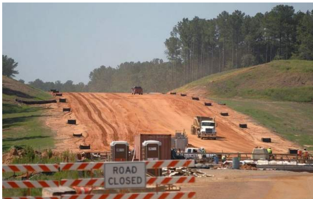
Work is ongoing at the new East Metro Parkway in Flowood, which is slated to connect Lakeland to I-20. The overall project, also touching Pearl and Brandon, is to be built in several phases. The portion in Flowood should be open in about a year. / Joe Ellis/The Clarion-Ledger
